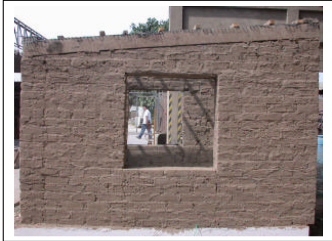
Figure 26 Model 2 South Wall, plastered side. The wall shows only small cracking with one vertical crack at the left wall intersection. See the sliding of the base at the right lower corner.
