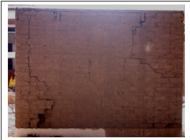
Figure 27. Model 2 West Wall. The right hand side without plaster shows cracking at mid height. The left plastered side shows damage at the lower part because the sliding of the North Wall.
