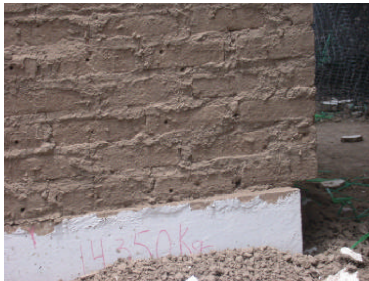
Figure 23. Sliding of the base in the North wall.
