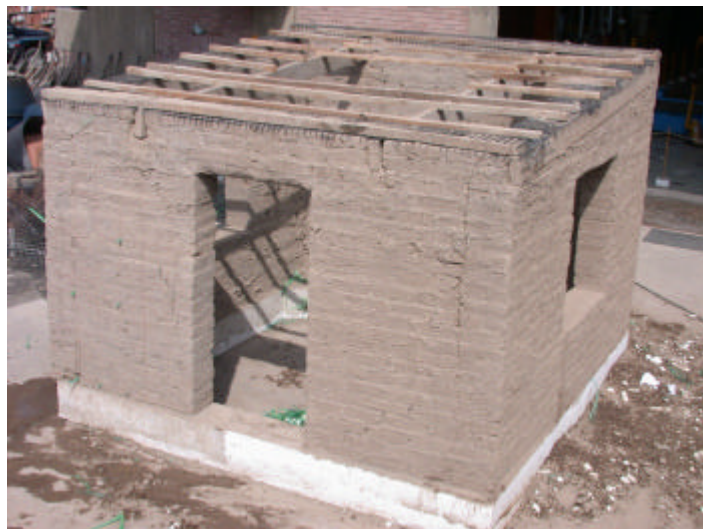
Figure 24. Model 2 after removing the plaster and the polymer mesh. The East and North wall shown here present only small cracking.
