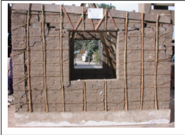
Figure 19. Model 1 South wall, without plaster. Damage is widespread but greater at the lintel level
