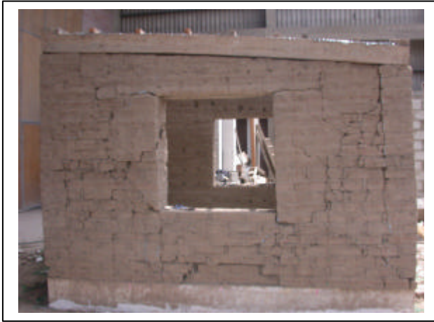
Figure 25. Model 2 North Wall without plaster. The wall is completely cracked after the test with more extensive damage in the left hand pier.
