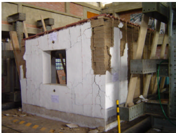
Figure 18. Model 1 after testing, view of north wall.
