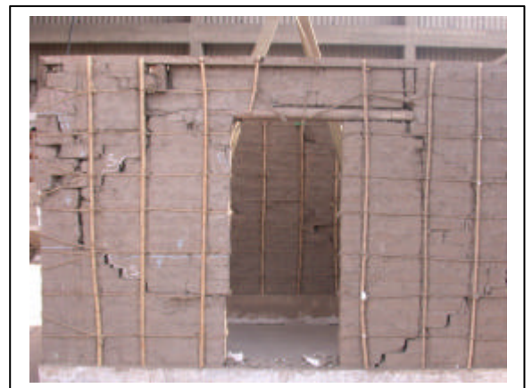
Figure 22. Model 1 East wall, The left side without plaster. Show greater damage than the right side
