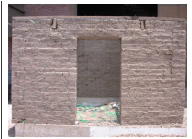
Figure 28. Model 2 East Wall. Only small cracking appear on this wall. The sliding can be seen at the lower left corner and a vertical crack in the right side.
