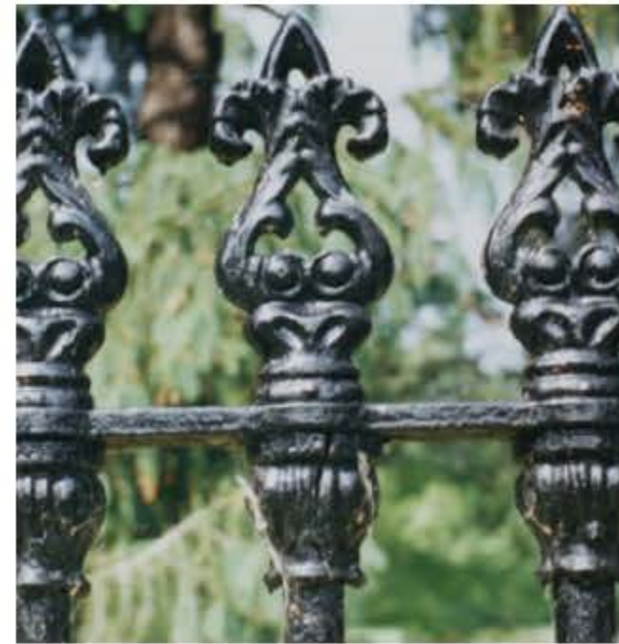
Typical fractured metal casting. Neglect of these deficiencies will lead to deterioration of adjacent elements
