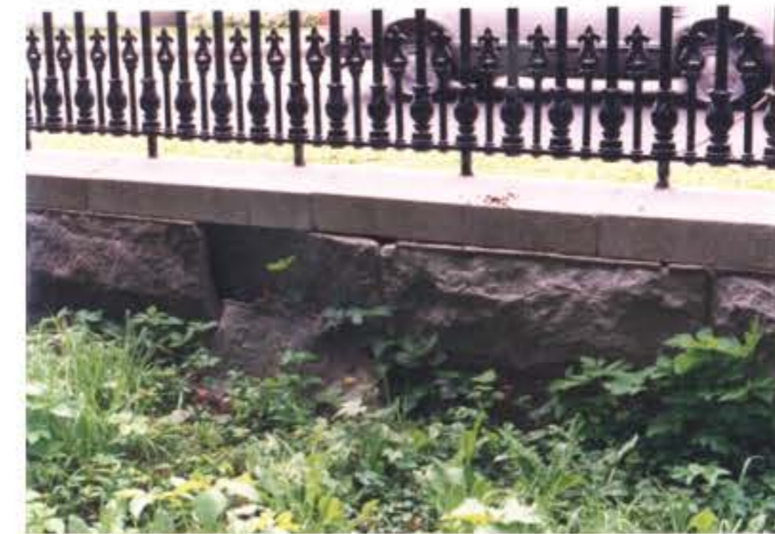
Typical failure at low masonry wall, Muckay Street.
