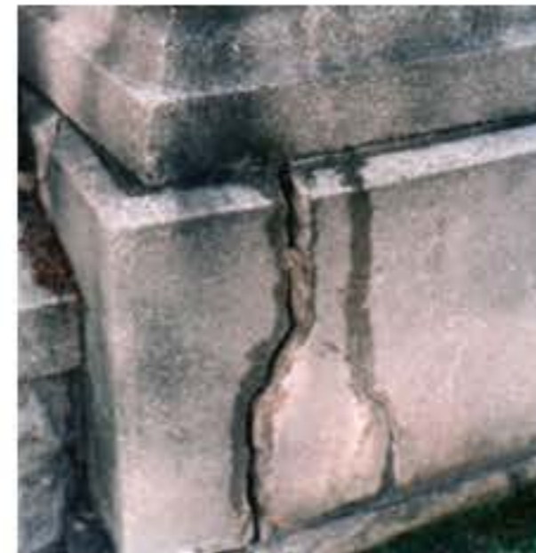
Typical Vertical Fracture at Base of Masonry Pillar
