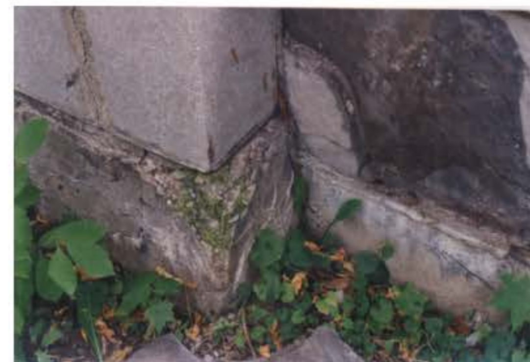
Typical spalled concrete at top of foundation
