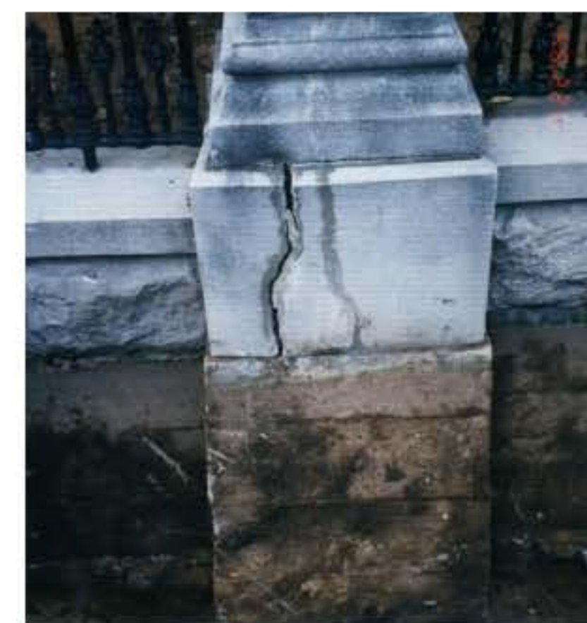
Typical cracked pillar base, partly caused by movement in foundation below
