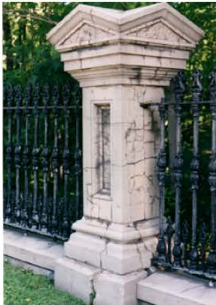
Typical fractures at masonry pillar (1933 Section).
