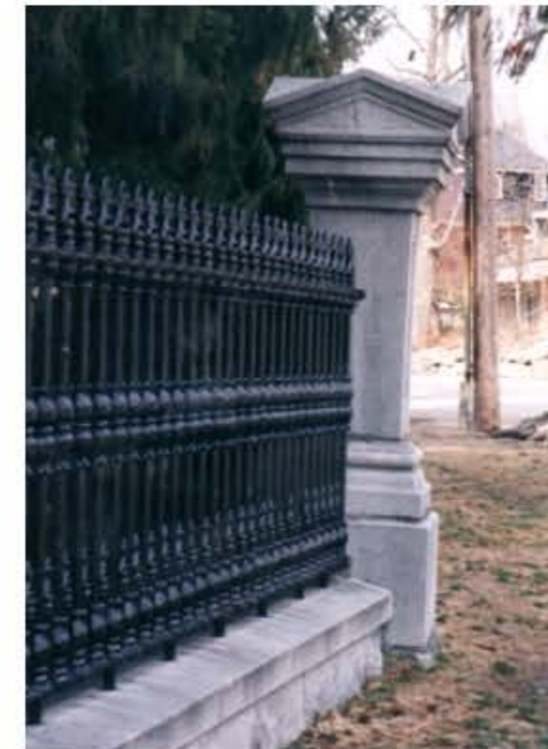
Fence assembly out-of plumb at section 1935
