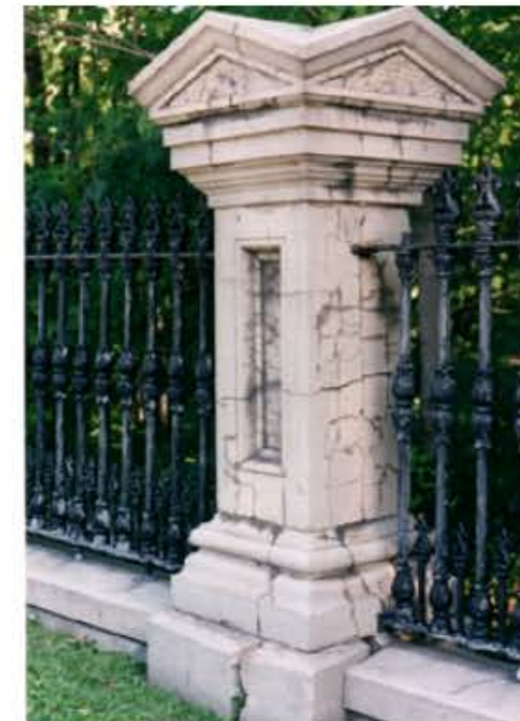
Typical fractures at masonry pillar (1933 Section).
