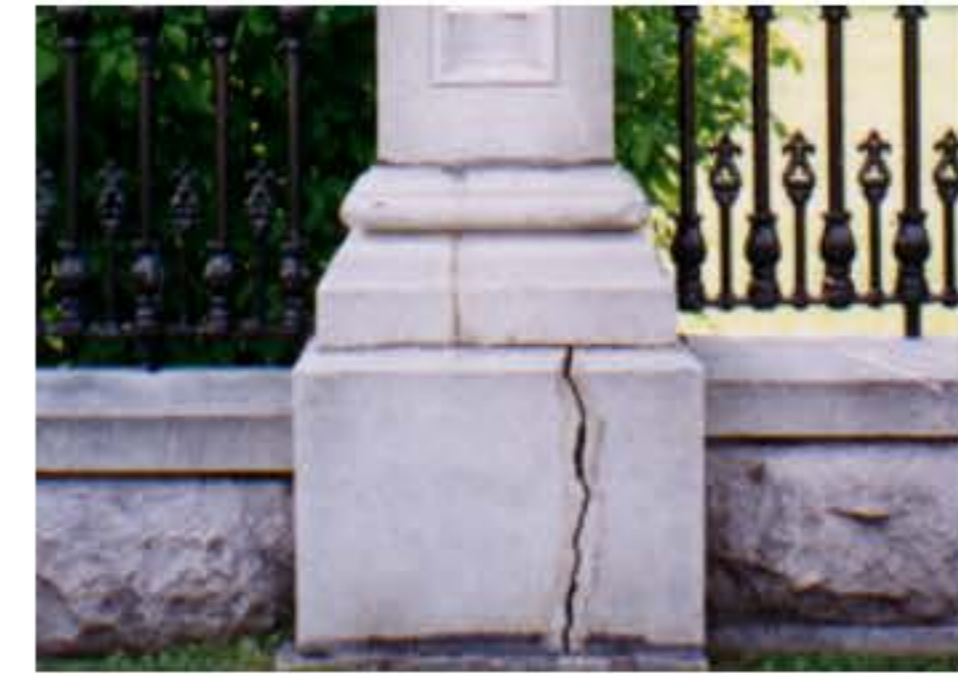
Typical Vertical Fracture at base of Pillar 144, caused by AAR-induced expansion in low wall adjacent, and in the foundation below
