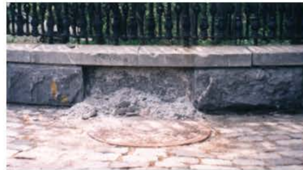
Typical failure at low wall
