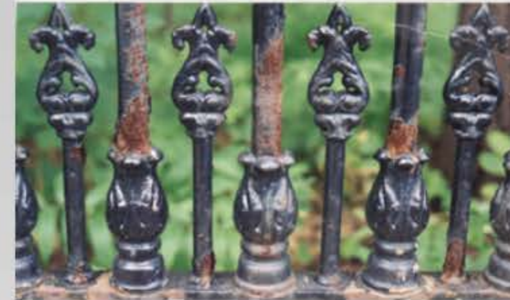
Typical corrosion at non-galvanized 1936 section
