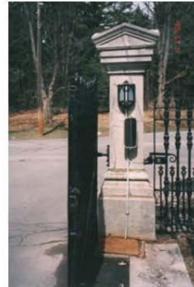
Surface-mounted electrical conduit at Prince Anne Gate :
