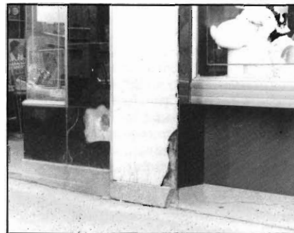
Snow removal equipment and lack of preventative maintenance demonstrate the vulnerability of structural glass at sidewalk level.
